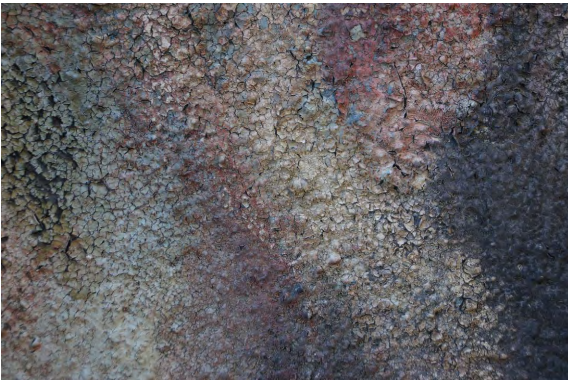
Detail showing breakdown of the paint binder – first stage of paint degradation eventually leading to cracking and loss of adhesion.
